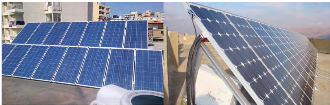
Figure 3: two PV projects installed by CEDRO
